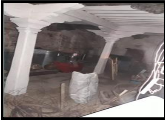
Figure: 16 (author) store room - wooden columns supporting the beams .mud roof covered with wooden planks.
