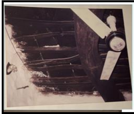
Figure: 10(author) Dhabi- wooden beams, rafters, planks above that mud moulds are placed with proper ramming with wooden mallet.
