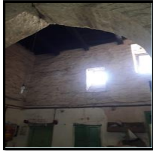
Figure: 21(author) Placement of ventilators at varying heights so that enormous light admits inside the kitchen, ventilator sill made inclined to disperse light below.
